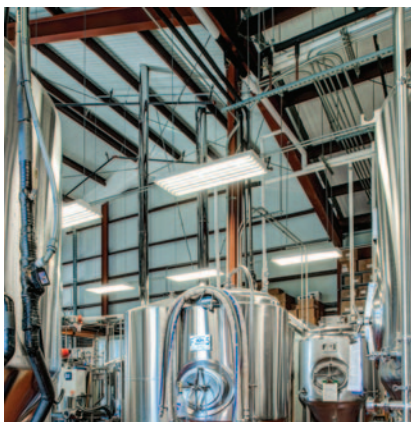
A brewery, rebuilt after a fire, used 2 HR fire-rated panels supplied by EcoSteel.
