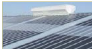
Solar Energy System
